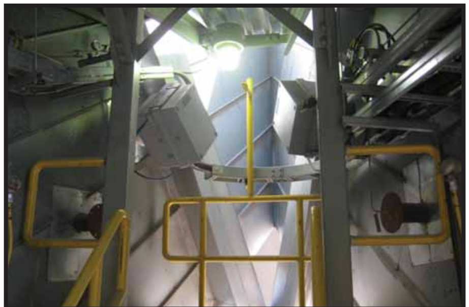
Probes allow sample process gas leading to the stack to be pumped to the analyzers
