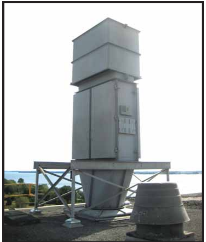
Finish Mill B exhaust silencer
